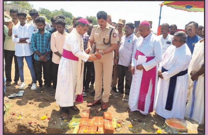
Laying of Foundation for 'Blessed Soosainather Alcoholism De-addiction Centre' at Celsini Colony, Caldwell Colony parish (19.03.2023)
